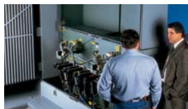
COOPER Power Systems
